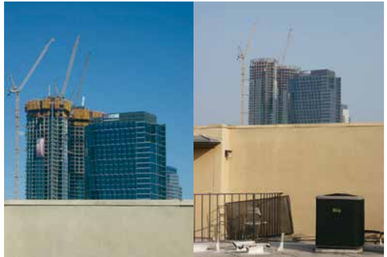
Figure 7. The luxury condominium building Century Plaza goes up near the intersection of Constellation Boulevard and Avenue of the Stars. Left: My view on July 4, 2020, with a celebratory five-story Stars and Stripes and the working platforms and third crane still in place. Right: Two months later, the concrete skeleton of the top floors is finished and the working platforms and third crane have been removed.
